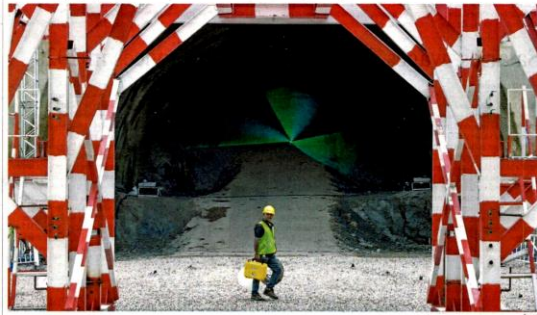
VIABILITY MATTERS: A 2019 file picture of a worker crossing the entrance to a tunnel under construction in Dungen for the ECRL. Several rounds of talks are expected between Selangor and Putrajaya before any final decision on the ECRL alignment is made.
